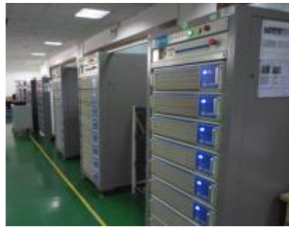
100V/100A Aging 100V/100A 老化設備
