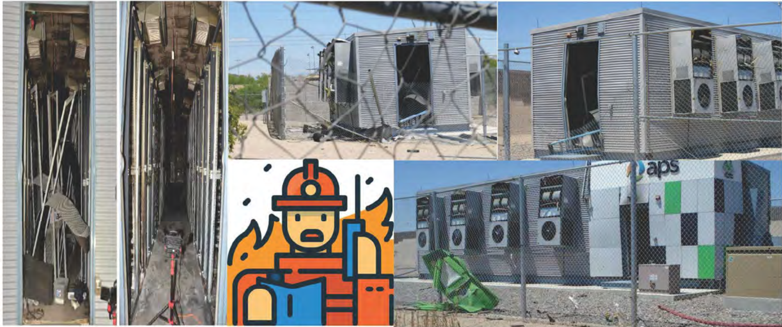
資料來源: McMicken Battery Energy Storage System Event Technical Analysis and Recommendations
