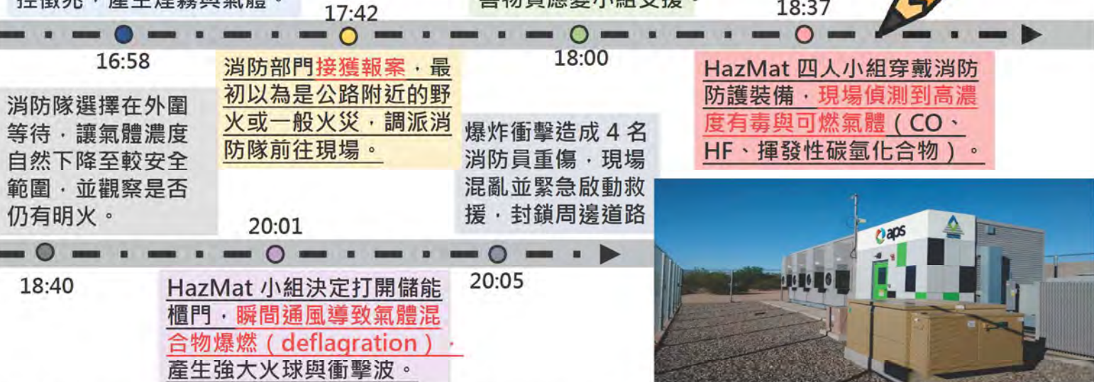
資料來源: McMicken Battery Energy Storage System Event Technical Analysis and Recommendations
